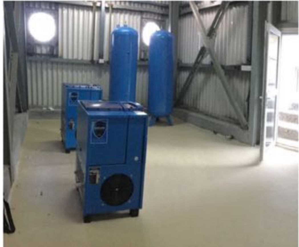
View of the ILMT compressor room
