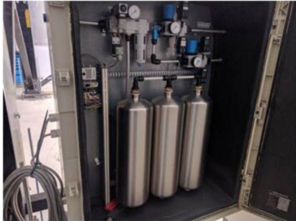
Pneumatic air control system in the ILMT main dome building.
