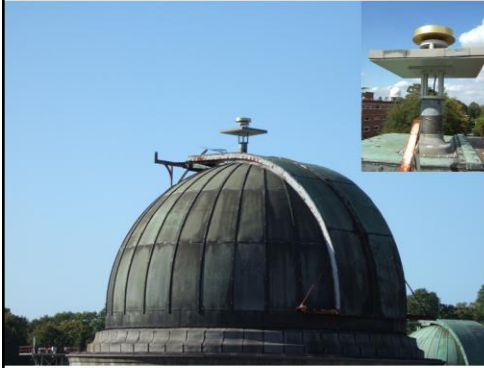
ROB GNSS antenna on telescope dome
